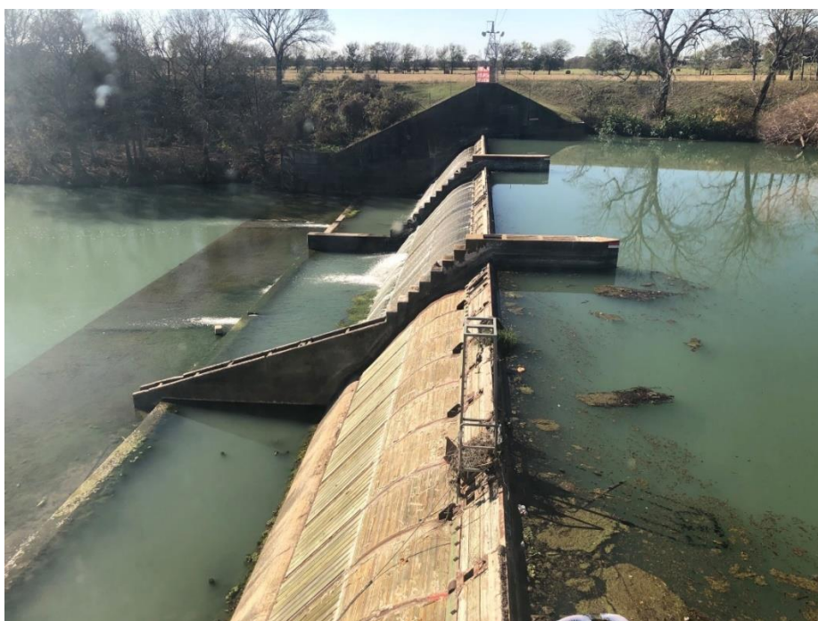
Figure 2-2: Nolte Dam Headwater and Tailwater Levels (view from control room)
